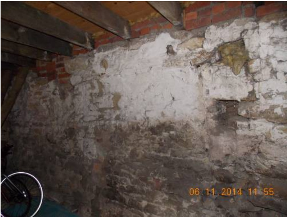
Timber lintel indicating blocked opening
